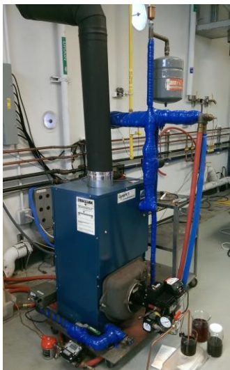
Image 2. Dunkirk residential boiler and Carlin fuel oil burner apparatus.
